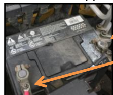
Ground connection (Black)
